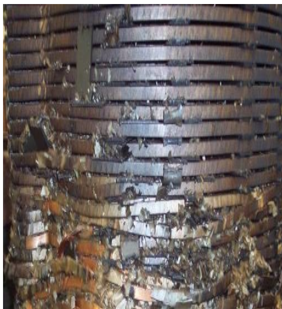
Figure 1. Power transformer exploded without preventive maintenance
