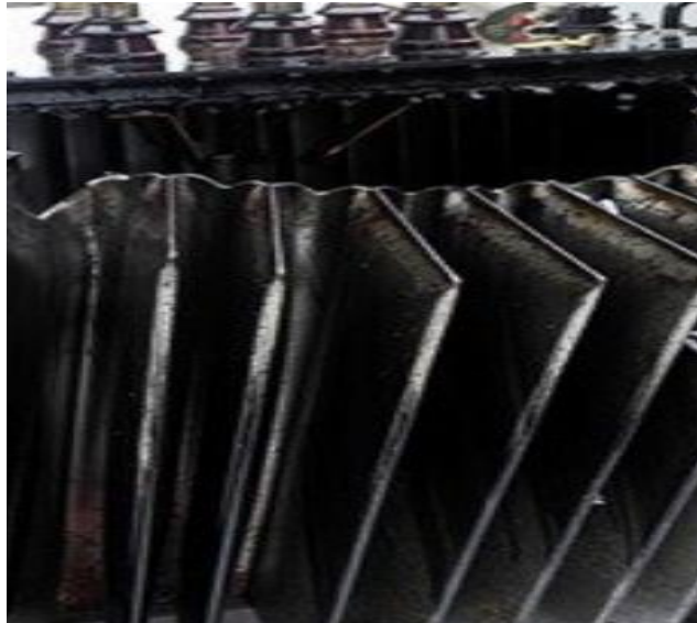
Figure 4. Transformer tank fault
