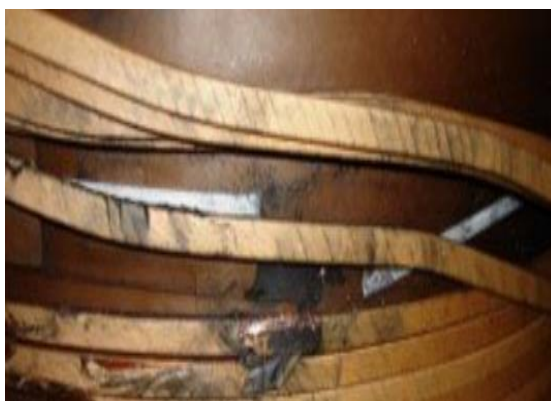
Figure 2. A short-circuit fault in the windings due to the tension and radial forces
